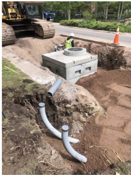
New electrical vault
