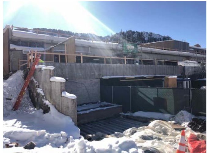
Brick & existing steel structure removal completed at the precast beam over the garage entry.
